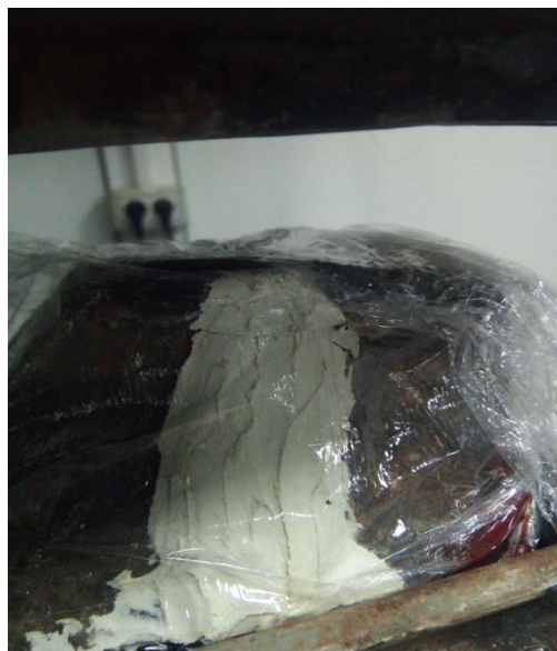
Fig. 2. Testing the resistance of the epoxy material in a superficial total crack
